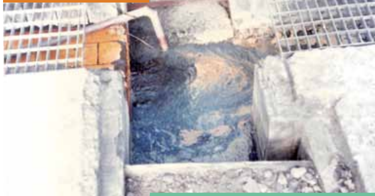
A drain flowing with effluent from a chemical production facility
