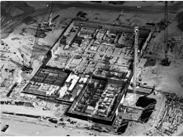
Figure 6.4. The Mixed-Oxide (MOX) Fuel Fabrication Facility, under construction at the U.S. Department of Energy's Savannah River Site, South Carolina, 28 September 2008. 273 Source: U.S. Department of Energy
